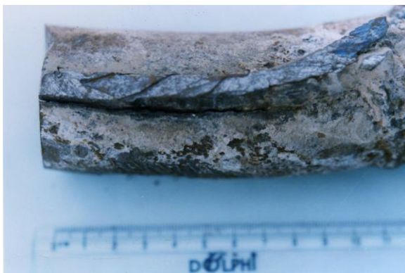
Fig. 3 Cracking in the tube
